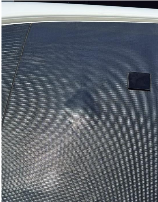
Fig. 10 - Trapped air causing visible deformation
