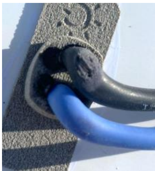
Fig. 13 - Insulation damage caused by sliding the panel over an unprotected rough surface
