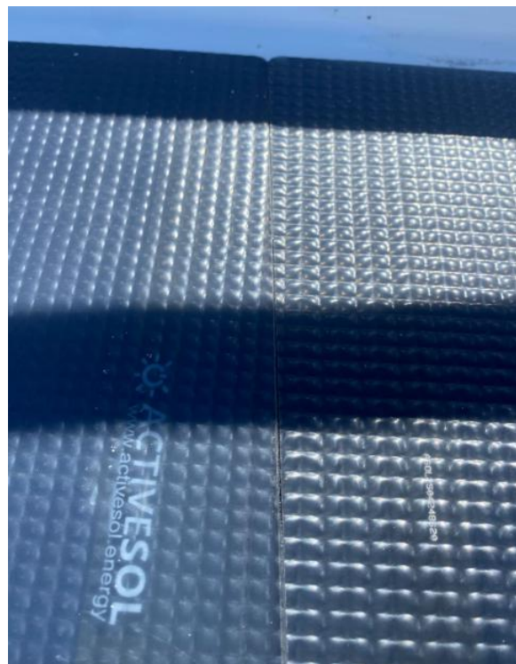
Fig. 11 - No expansion joint left between adjacent panels
